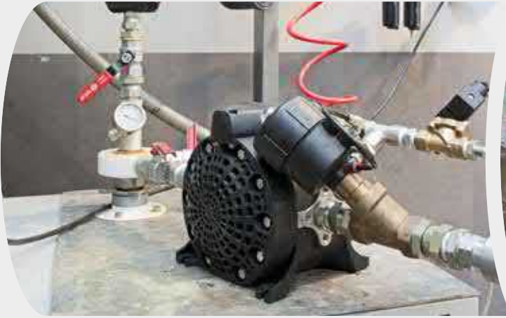
Cement additive dosing.
