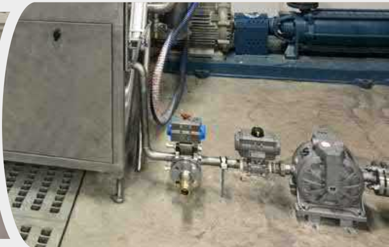
Chemical products dosing.
